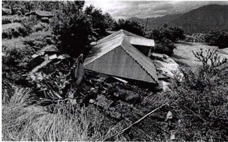
Figure-6: Showing damaged house
