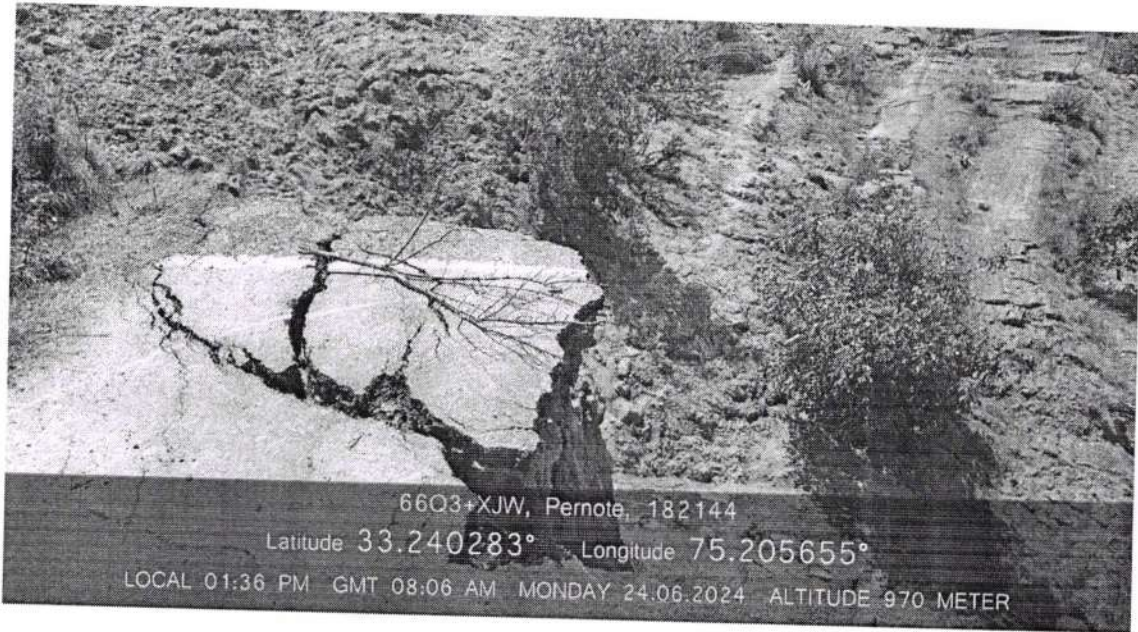
Pic-4: Damaged Parnote-link Road at Parnote.
