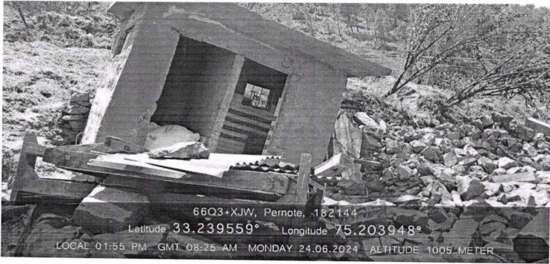
Pic-7: Damaged structures.
