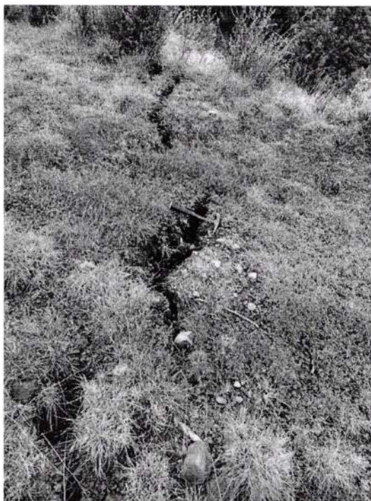
Figure-10: Showing transverse cracks developed near crown
