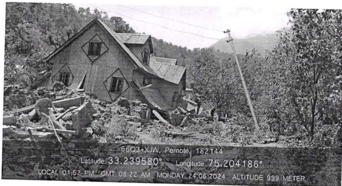
Pic-5: Damaged Houses.
